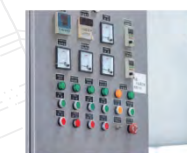
Power equipment testing
