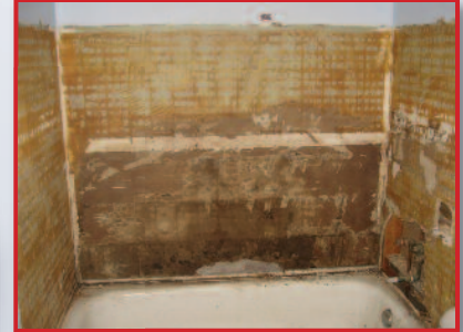
Wet drywall behind removed bathtub tiles
