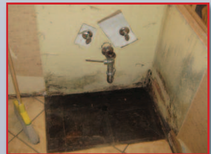
Locate moisture or water damage
